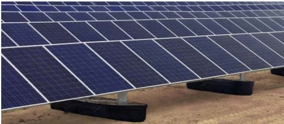
Figure 3: Example photo of a ballasted solar PV array on a landfill.
